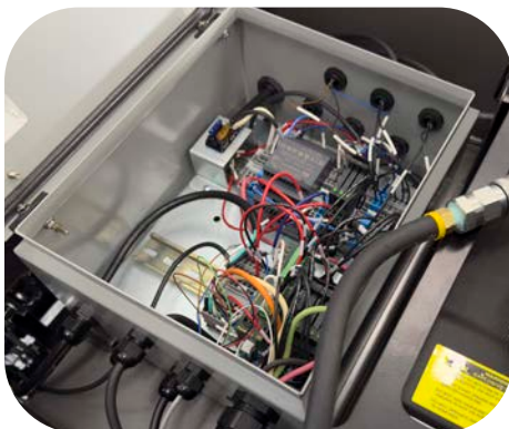
Larger Accessible Electrical Box
